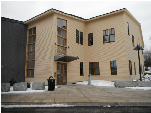
The redesigned and reconstructed new side entry and plaza to the MCA.
