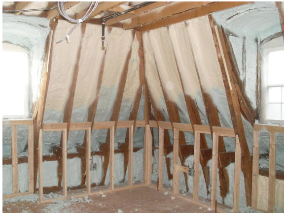
New insulation in previously un-insulated walls and Mansard roof on 3 rd floor
