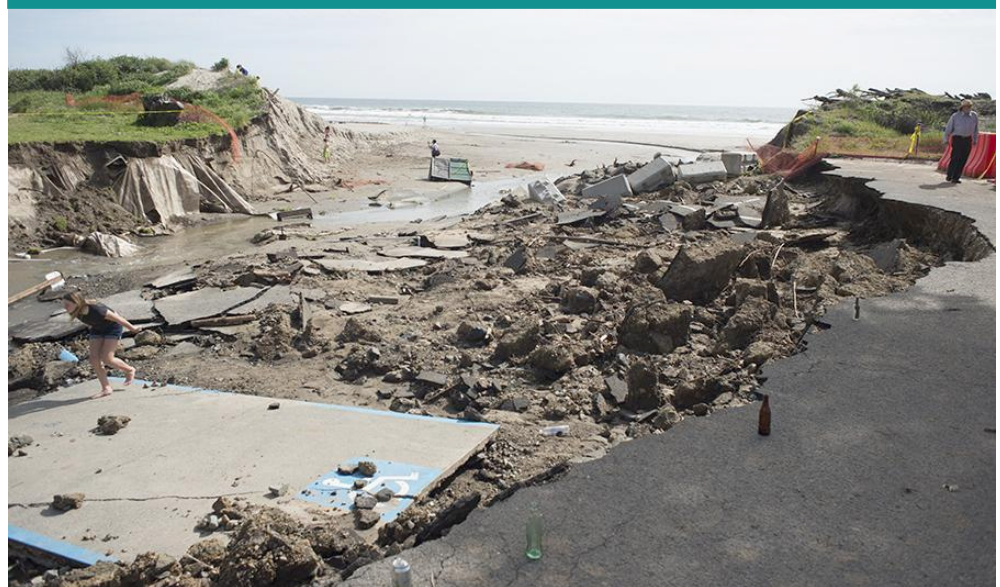
Stinson Beach parking lot closed in 2018 after a storm caused part of it to fall into the ocean (Figure source: David Briggs, The Point Reyes Light).
