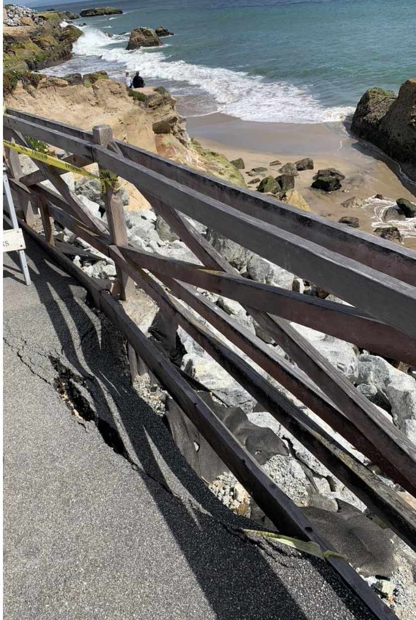
Figure 2-2 Erosion Incident on West Cliff Drive: 2019
